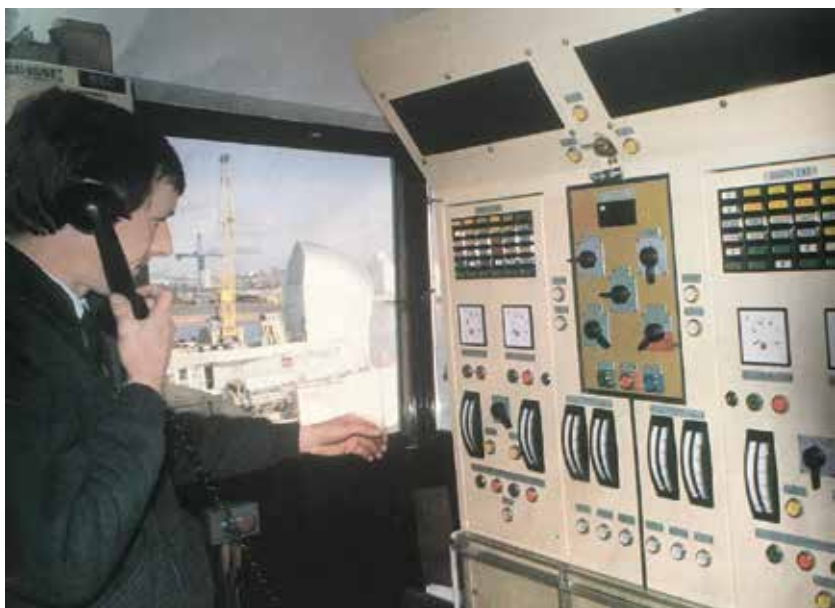
Fig 65. Control Room testing
